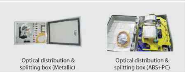
Network access point in building
