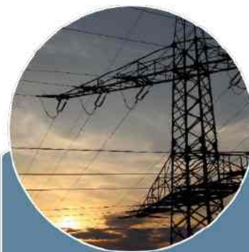
Overhead Transmission Line
