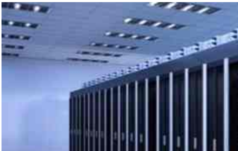
Data Center Cabinet
