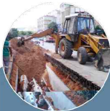
Underground Cable System
